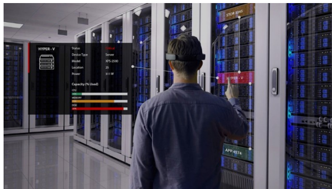
Figure 3 A data center operator wearing a small MARS headset in order to view the different components in a server
